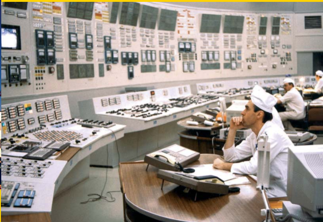
The operations at the Leningrad nuclear power plant are monitored in the control room. Photo: Norwegian Radiation Protection Authority
