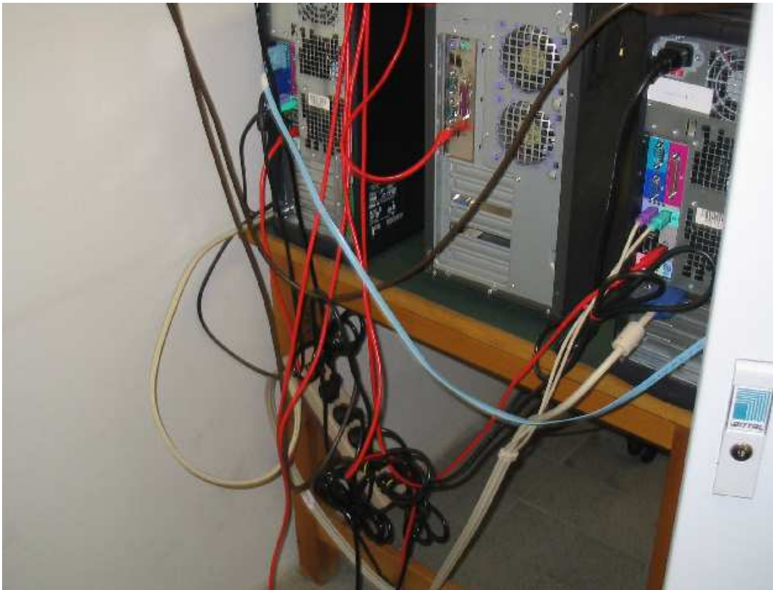
Figure 2.1: Don't do this. Power connectors should not be hanging in mid air, as this means they are stretched and can come apart, causing an accident. The red network cables should not be tangled and hanging like this.
